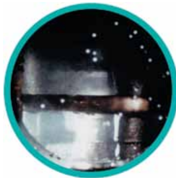
FIGURE 6-12: More than 60 seconds after start-up, oil level is well below normal operating levels - a condition that is an important factor in compressor bearing wear.
