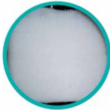
FIGURE 6-11: Five seconds after start-up, violent foaming action fills sight glass as refrigerant boils away taking the oil charge with it.
