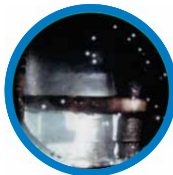
FIGURE 6-4: More than 60 seconds after start-up, oil level is well below normal operating levels - a condition that is an important factor in compressor bearing wear.
